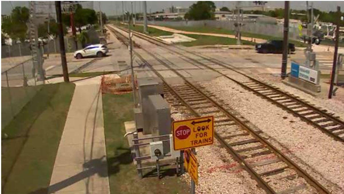
Railroad Crossings equipped with video surveillance
