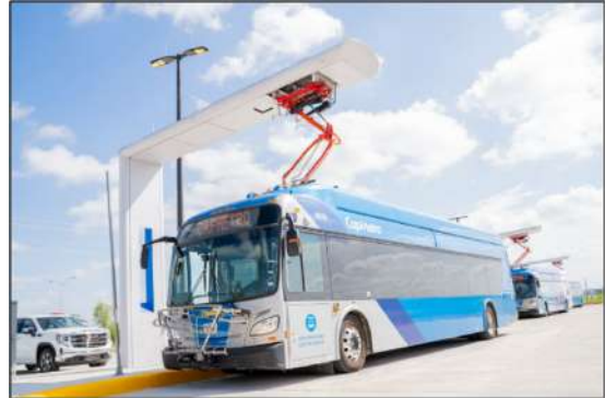
Bus and electric charging infrastructure
