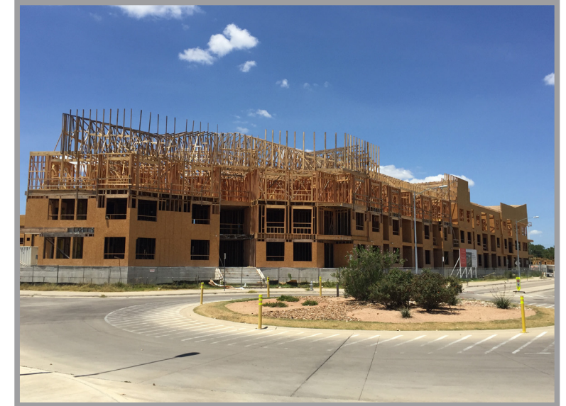
Mixed-use development, townhomes, and senior living is under construction on Alexander Street, 17th Street, and MLK Jr Boulevard at the station
